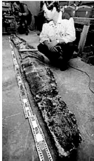
Fig. 1. A giant concrete chunk fell from the wall of a tunnel.
