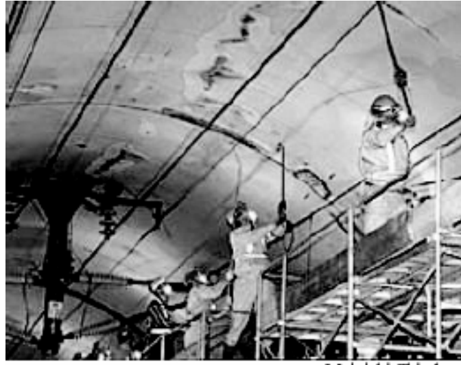
Fig. 2. The JR West Company inspected 142 tunnels and found 2,049 points with faults.
