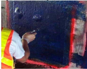
Figure 4. Intentional Delaminations on FRP Laminates.
