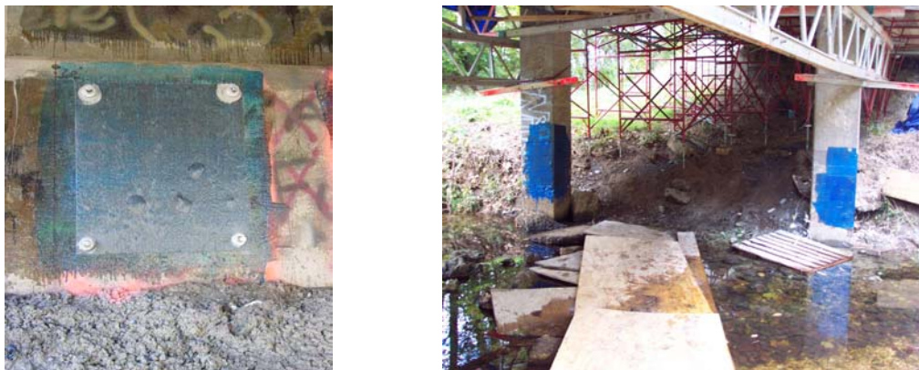
Figure 8. CFRP laminates with delaminations on south abutment and north bent
