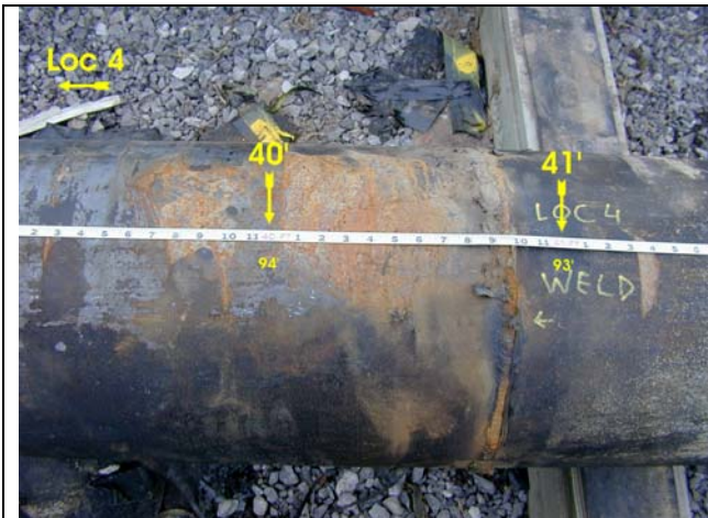
Figure 10. Dis-bond and minor surface corrosion over 180° between 40' and 41'. Similar areas corresponding to anomalies I, J & K (Figure 12) from Location 4 were noted between 35' and 39'. The weld is visible just before the 41' mark and corresponds to the typical weld signal @ "L" in Figure 12.
