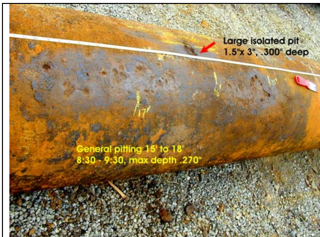
Figure 4. Severely corroded area approximately 3 feet in length with numerous isolated pits and areas of general corrosion. Included in the section was a very larger isolated pit (marked by arrow at top right). See Figure 6 showing signal response from this area – 14 to 18 feet.
