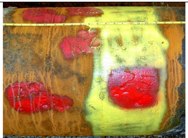
Figure 5. Isolated pitting and general corrosion 360° around the pipe and on either side of the weld. Yellow paint indicates area identified by GWUT; red spots were from smart pig data and were marked where they exceeded 50% of nominal wall. See Figure 7 showing signal response from this area – 16 to 17 feet.
