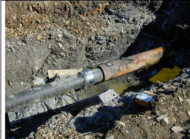
Figure 8. GWUT Tool position set-up for inspection of a cased road crossing. Casing end-seal has been removed.
