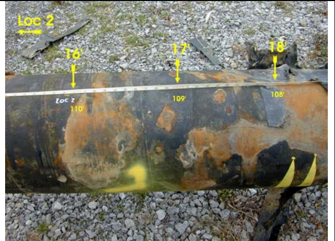
Figure 9. Surface corrosion delineates areas where coating has separated from the pipe. Good coating adhesive is represented by black areas remaining after stripping the coating material. Areas such as this indicating water migrating under the coating correlated with many of the signal anomalies.
