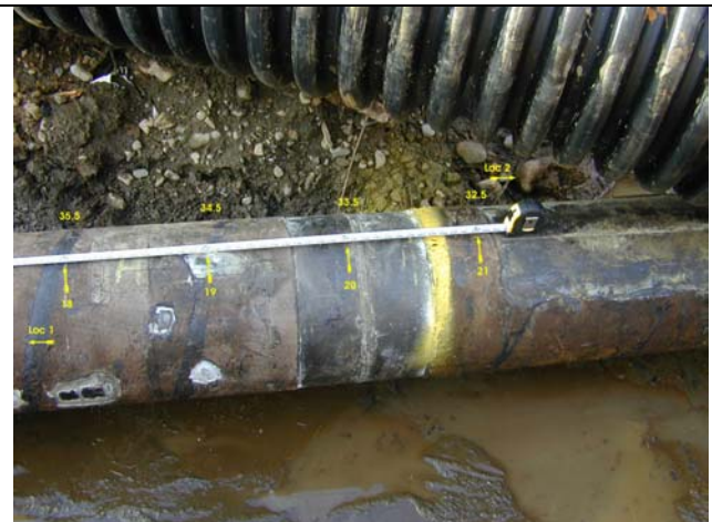
Figure 11. 18 to 21+ feet from datum @ Location 1 showing weld just past 20' and bare pipe on either side of the weld. Signal responses for the coating transition to bare pipe were present but at low amplitude from Location 1. From Location 2 the transition from bare pipe to factory wrap coating @ 34' (yellow band – right center) corresponds to the arrow marking an undesignated signal peak in Figure 13. Note coating patches missing lower left on pipe. Signal trace data representing this area is shown in Figure 13.
