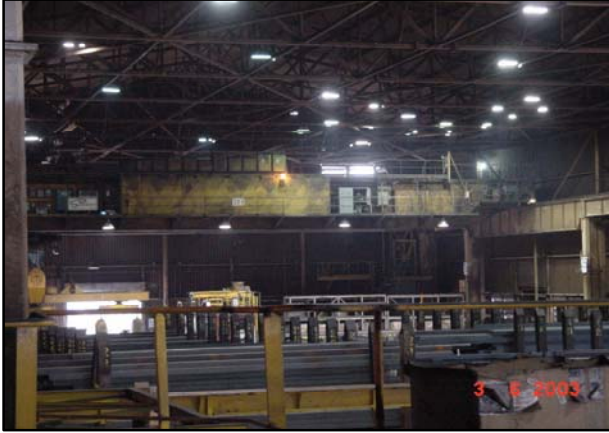
Picture No 3: 22 tons heavy service overhead crane
