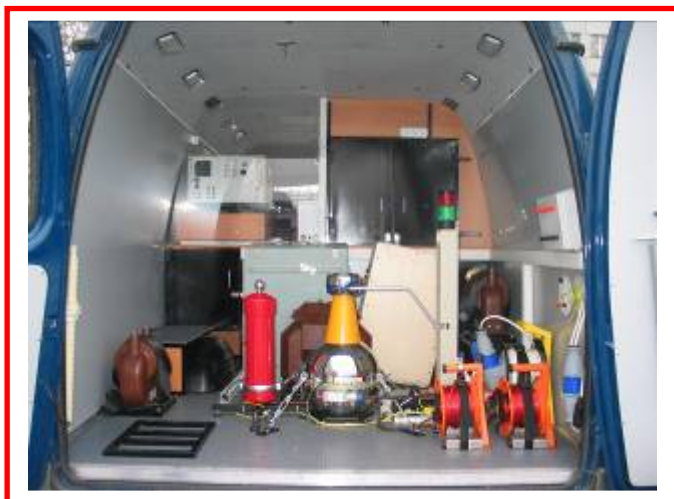
Fig.7. HV Equipment Compartment
