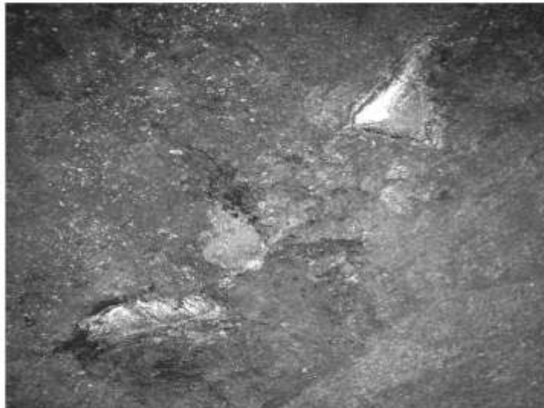
Figure 8. Internal defect on the heat exchanger cover
