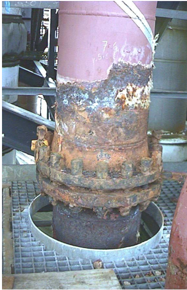
Figure 1. Picture of a steel pipe with external corrosion damage resulting from ‘Corrosion under Insulation’ (CUI)
