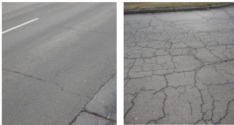
Fig. 2. Thermal cracking (left) and block cracking (right) on asphalt concrete pavements in Illinois.
