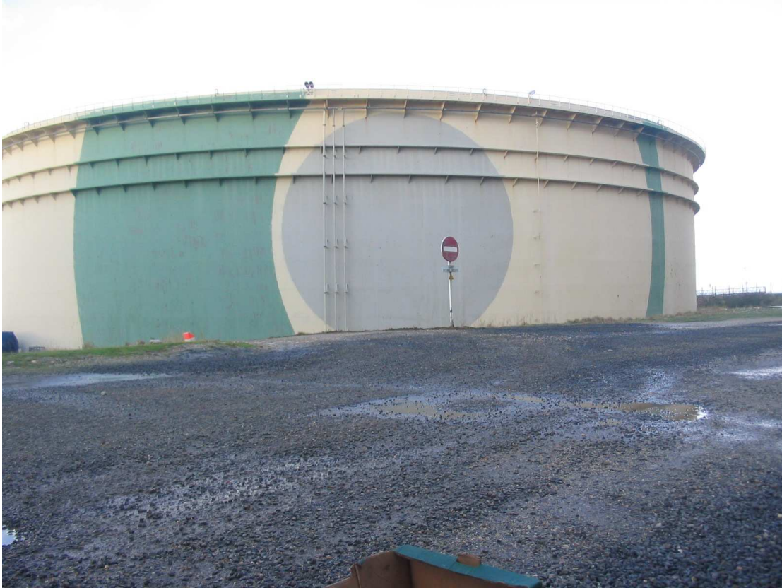
Figure 4. Large capacity above ground oil storage tank
