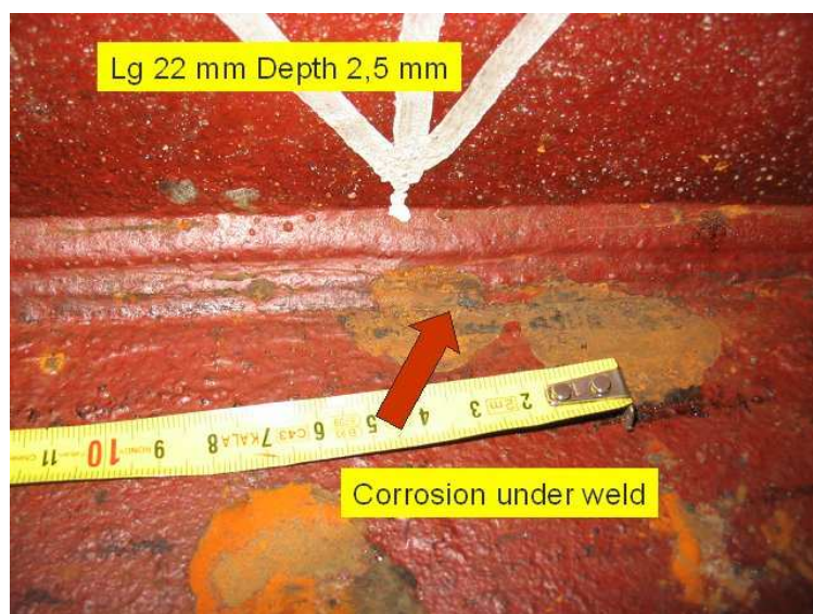
Figure 11. Localised corrosion under weld toe
