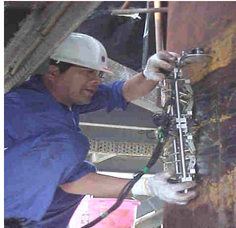
TOFD set up and D- scan image-showing defect on the weld
