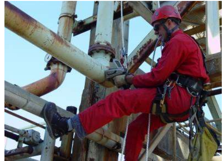
Handheld Thermo Scientific Niton XRF analyzer being used to inspect piping system
