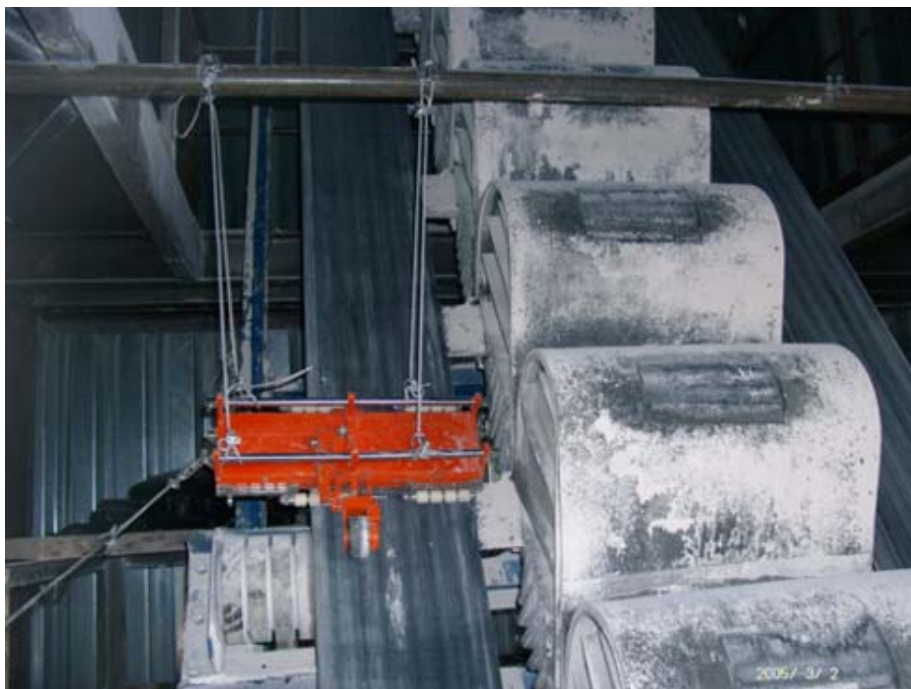
Fig. 6: The INTROCON scanner positioned on the Pocketlift conveyor belt.
