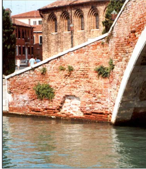
Figure 6 – Detail of local damage of S. Donato bridge
