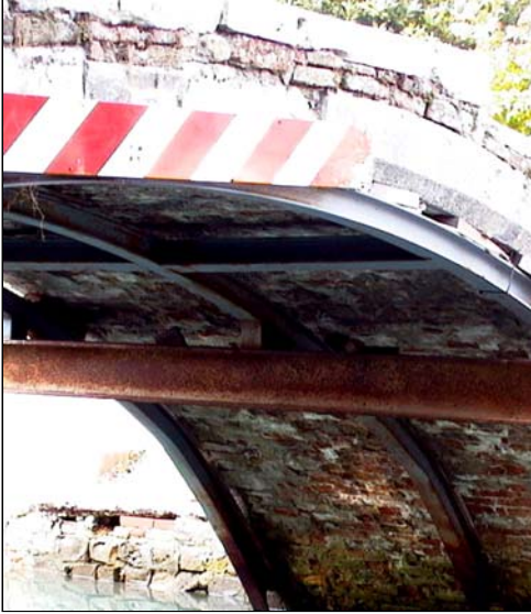
Figure 5 – Detail of local damage of Devil bridge
