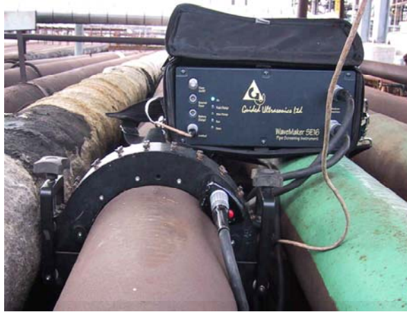
Fig 1. Solid transducer ring for 8 inch pipe and battery powered test instrument on site.
